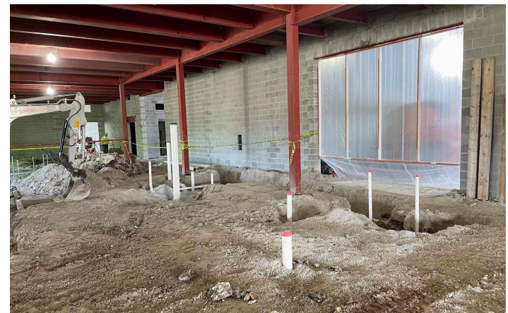
Underground, plumbing pipes are strategically placed to facilitate the flow of water throughout the building. These pipes will be concealed beneath the concrete slab on grade.
